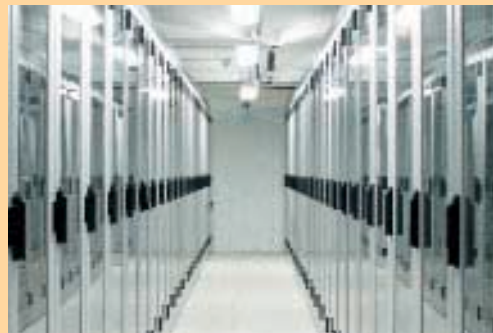
Just one Data Center alone contains 11 rooms with space for over 660 racks for a total of 26,400 servers.
