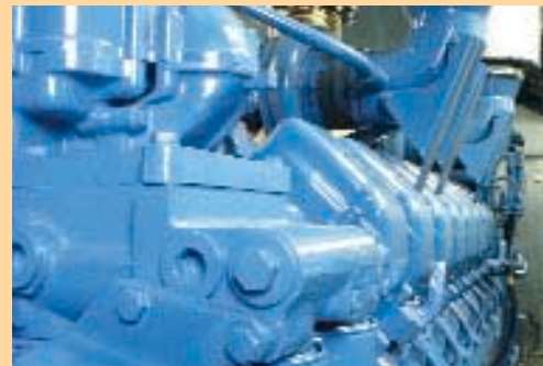
Powerful diesel generators supply constant, reliable power.
