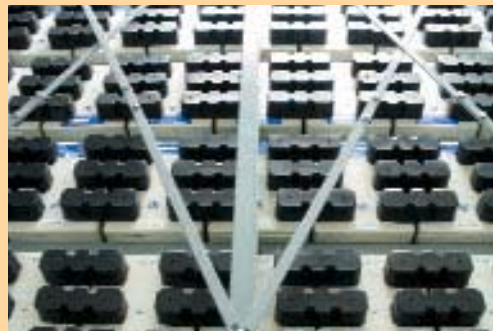
Lead gel batteries guarantee continuous power without interruption.
