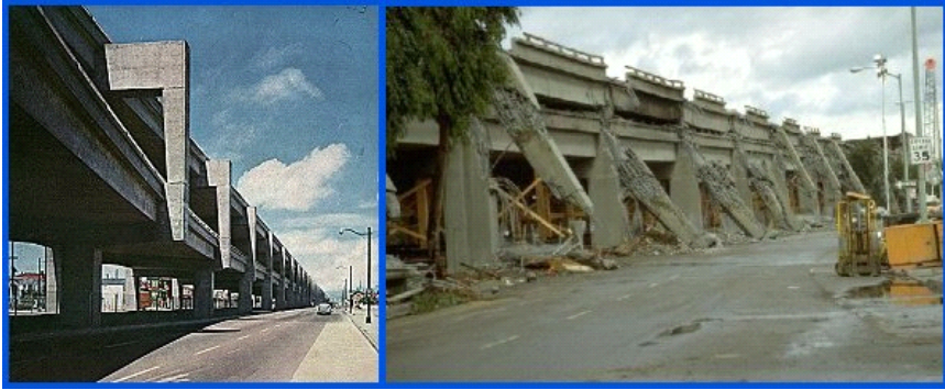
FIGURE 2.1 The Cypress Street Viaduct (left) before the earthquake of 1989 destroyed much of the structure (right), requiring its demolition. SOURCE: EBMUD Seismic Improvement Program. Available [on-line] at: http://home.pacbell.net/hywaymn/Cypress_Viaduct_Freeway.html
