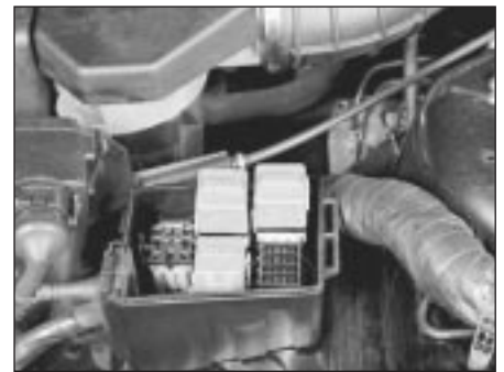
4.2 Engine compartment relays
